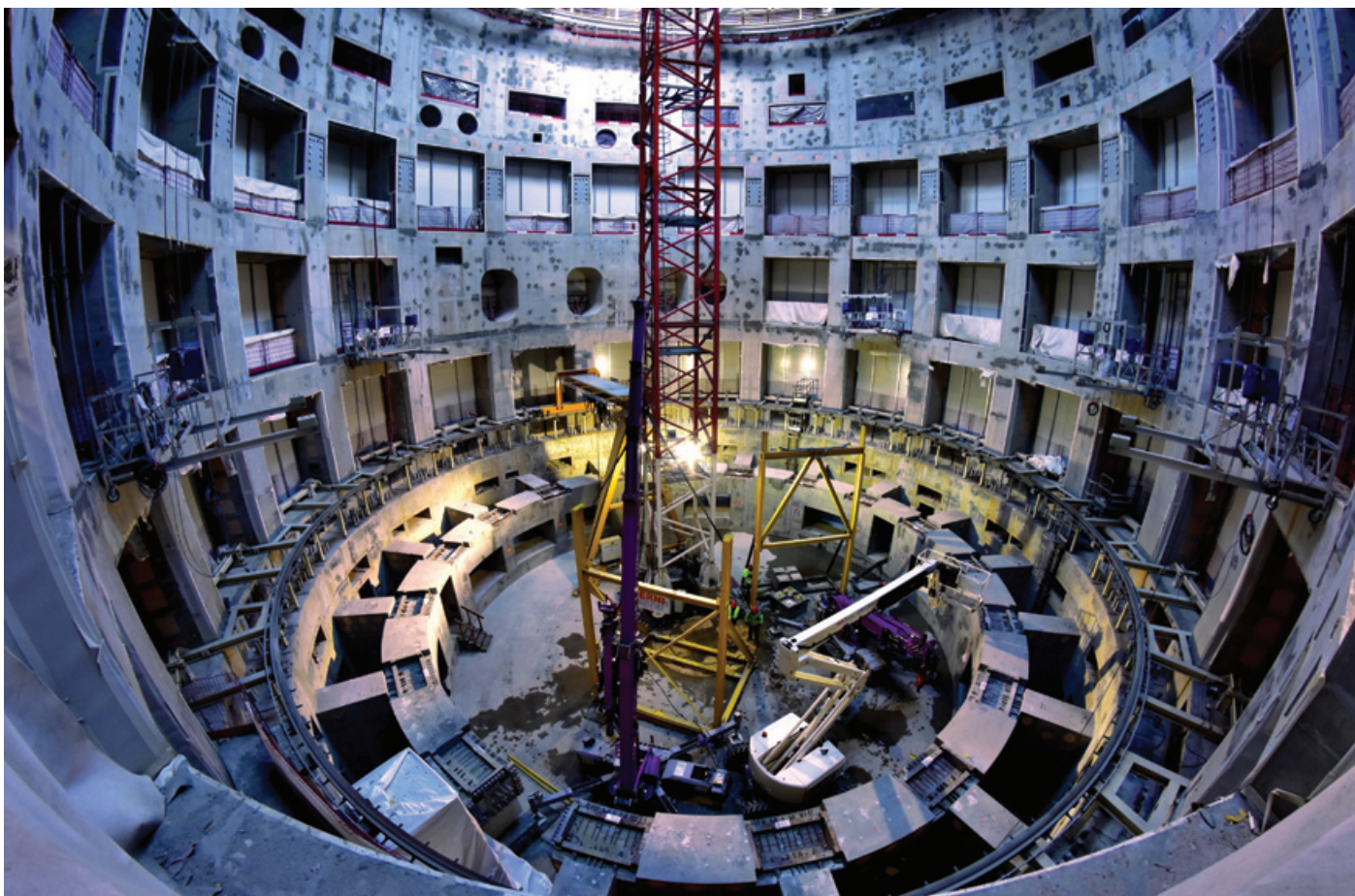
The 23,000-tonne ITER Tokamak will rest on a massive circular “crown” at the bottom of the bioshield. The openings in the cylindrical structure are for the different systems that need to reach into the machine: power feeders, vacuum pumping, heating, cryogenics, cooling water, diagnostics, etc. © ITER Organization.
