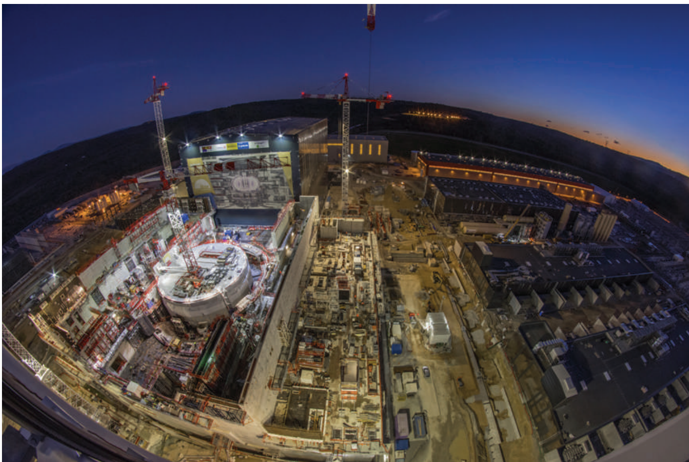
The heart of the ITER installation: to the left, the Tokamak Complex with the circular structure of the "bioshield", a 3-meter-thick steel-and-concrete cylinder that will enclose the ITER Tokamak; to the right, the installation's industrial facilities (power conversion buildings, cryoplant, winding facility, etc.) (December 2018). © ITER Organization.
