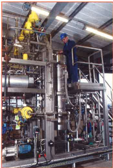
Figure 4 - View of the reactors in the Thomas Swan and Co. Ltd. scCO 2 plant in Consett, Co. Durham (UK). Photograph, courtesy of Thomas Swan and Co. Ltd.
